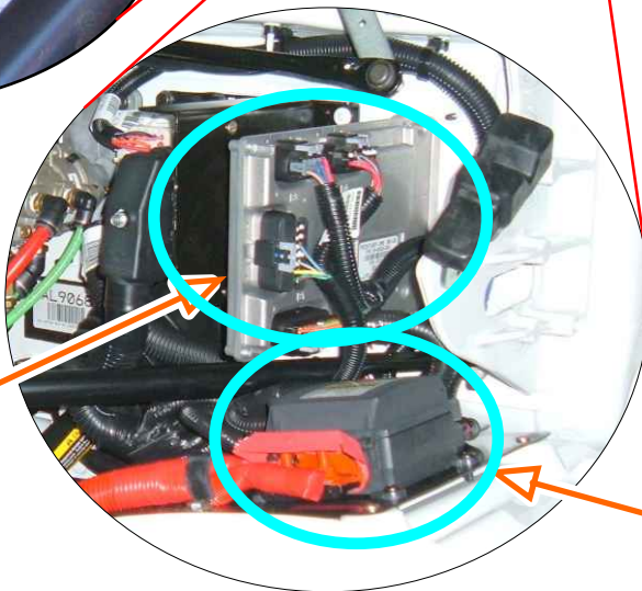
Power Distribution (Module 285 PDM)
